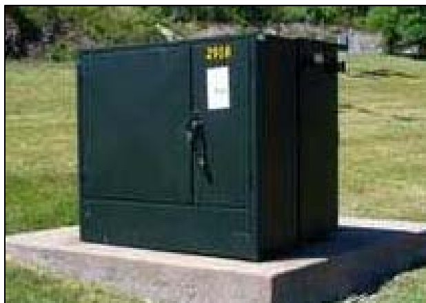
Figure 24: Pad-Mounted Distribution Transformer
