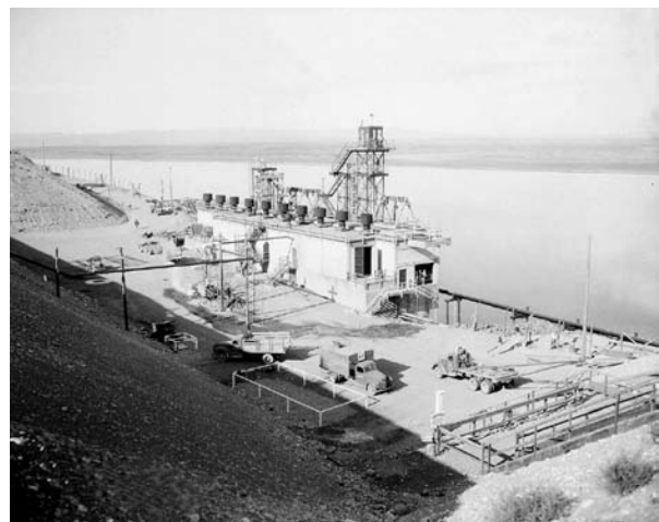
Columbia River Water Pumping Station
